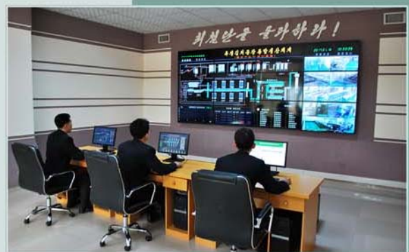
The general control room.
